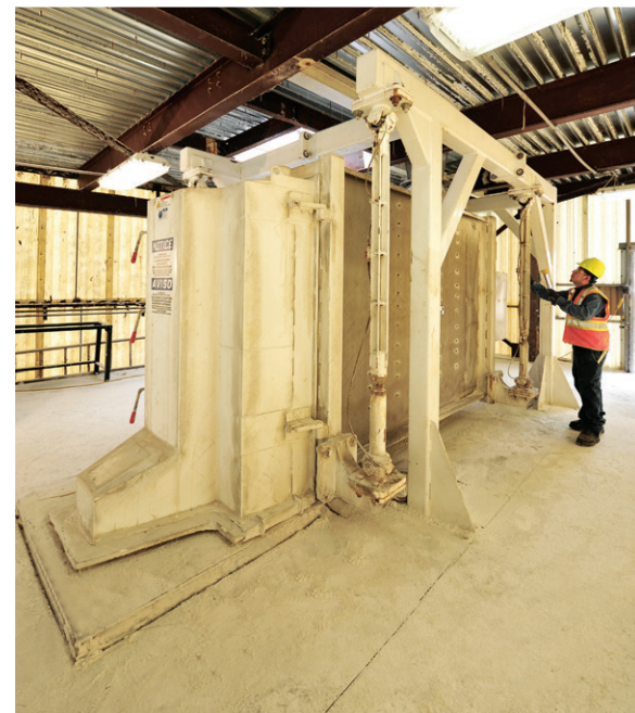
Figure 4: Rotex Minerals Separator Installation
